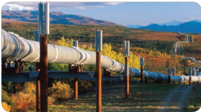
Figure 6: Because of their remote locations and distance from infrastructure utilities, pipeline applications often rely on gas-powered actuators to automate large isolating ball valves.
